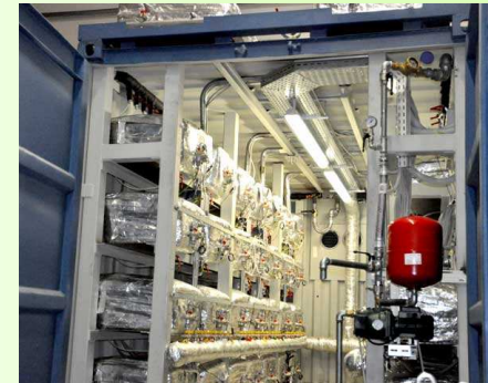
Image: Interior view of first generation ECAT 1 MW Plant. Note the racks are built of smaller ECAT kW units in parallel. Image from http://ecat.com or http://ecat.com/ecat-products/ecat-1-mw/ecat-1mw-pictures
